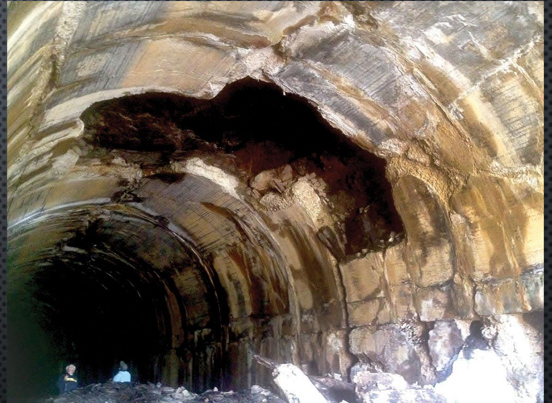
Figure 3: Cracking due to freezing and thawing over time [5]
